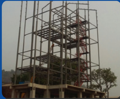
Nigeria - Unikem Boiler Structure
