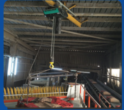
Holcim Cranes - Chekka
